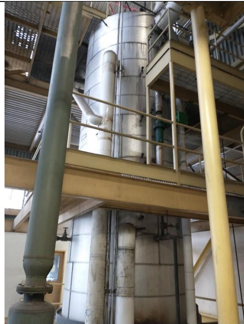
Figure 2. Hot Lime Softening system at Energy Plant requires make-up water.
