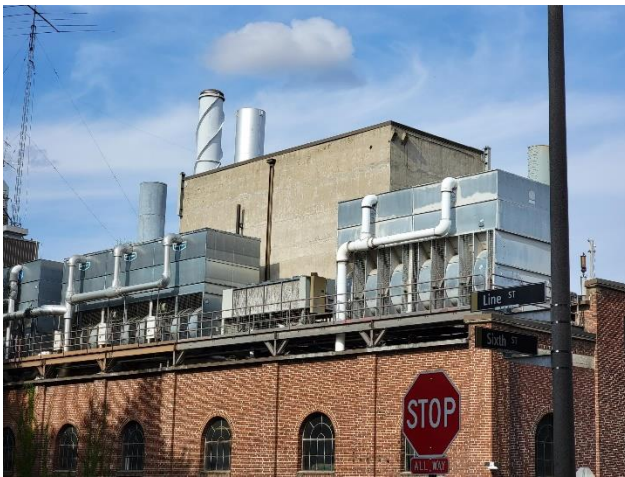
Figure 1. Cooling towers at Energy Plant.
